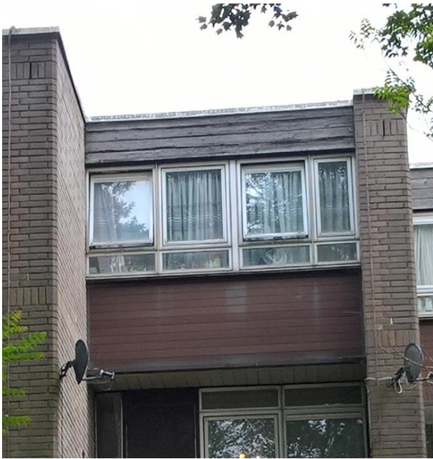
Flaking & Peeling paintwork to timber cladding to maisonette
