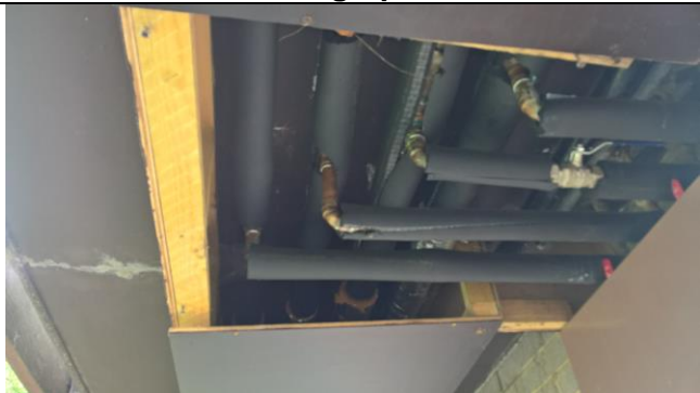
Exposed service pipes serving flats.
