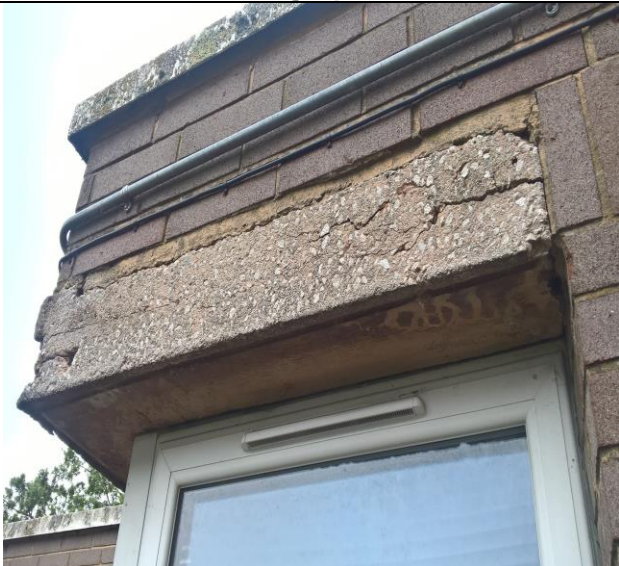
Cracked concrete to lintel-beam
