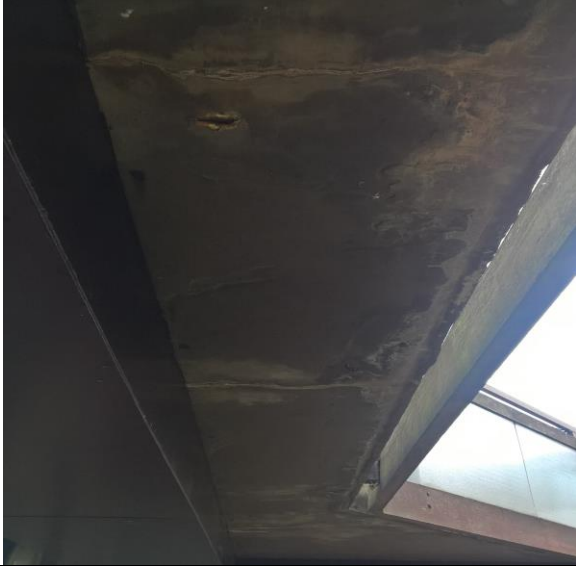
Cracks on communal balcony soffit and service duct to full length.
