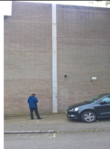
Boarded up window in flank wall –Flat-12
