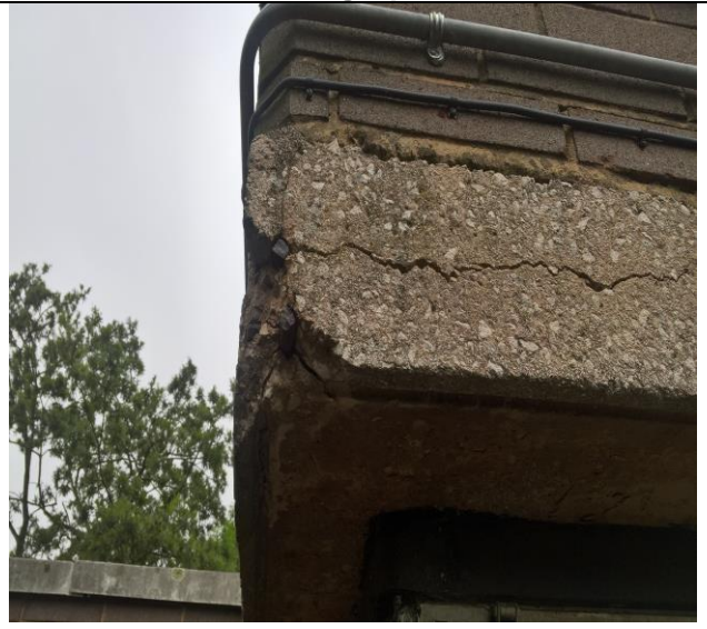
Corroded and exposed reinforcements to lintel-beam due to detached concrete
