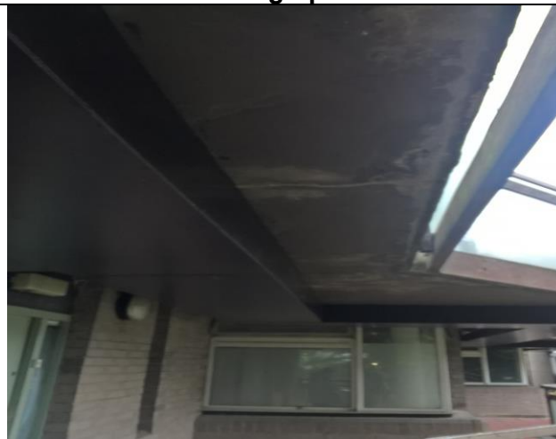
Horizontal cracks & water stains in the soffit
