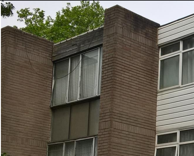
Peeling & Flaking paintwork to timber cladding (flat-22)
